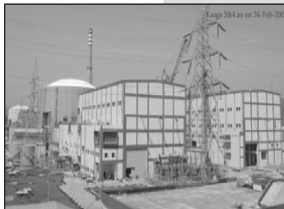
Kaiga Atomic Power Project 3 & 4
