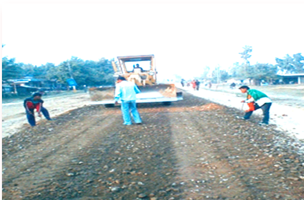
The Terai Road Project in progress. Courtesy: Observer Research Foundation's Special Report on India's Development Cooperation
