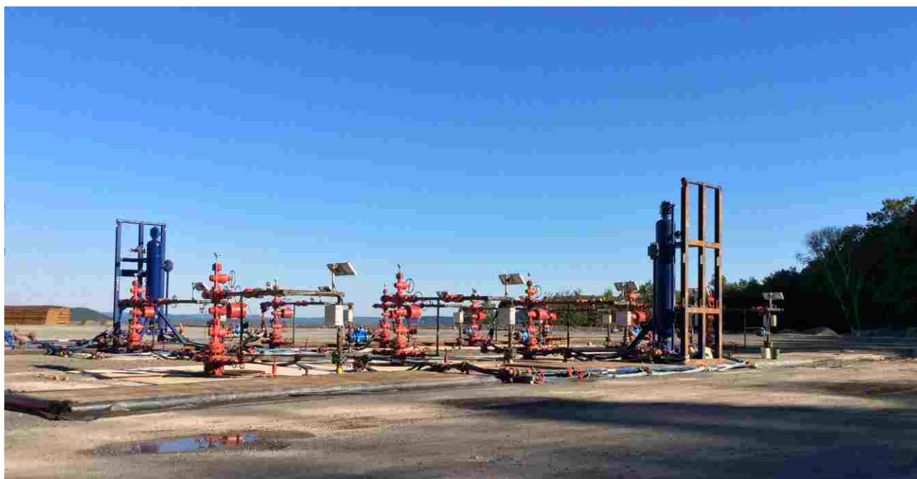
A typical well pad with multiple shale gas wells in the US
